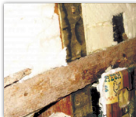
Figure 5 Urea Formaldehyde Foam Insulation
